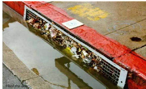
A clogged catch basin in Los Angeles.
