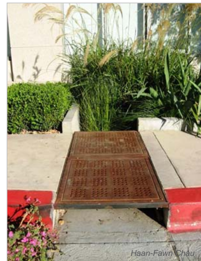
A curb cut that directs water from the street into a bioswale. 1100 S. Hope Street in downtown Los Angeles.
